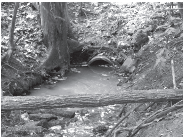
Figure 3.5: Stormwater pipes can deliver surges of water that is typically polluted to impacted natural areas
